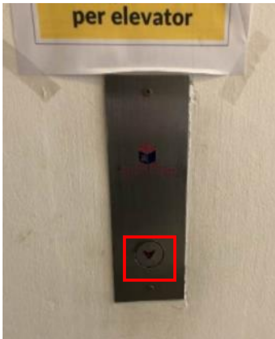
Figure 2-10 Core 4 Test Apartment block Lift Call Button
