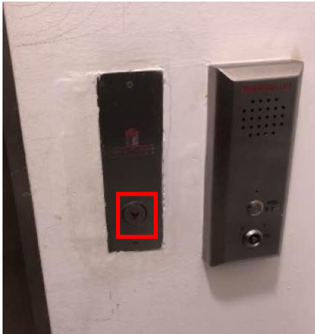
Figure 2-1 Core 4 Test Apartment block Lift Call Button
