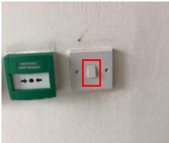
Figure 2-6 Core 4 Test Apartment block Lobby Door release button
